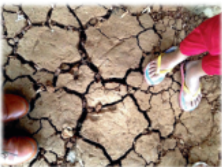
The floor of the church building – need funds to cement it
